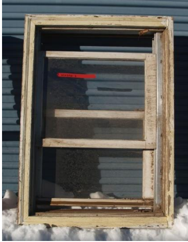
Window 7 Double hung window, retrofitted with new slider hardware 29" x 37.5" From 401 E. Geneseo St.
