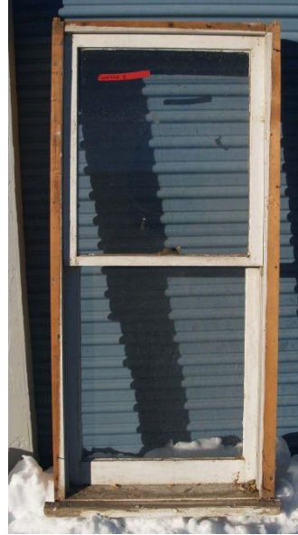
Window 8 Double hung window, retrofitted with new slider hardware 26" x 57.5" From 401 E. Geneseo St.
